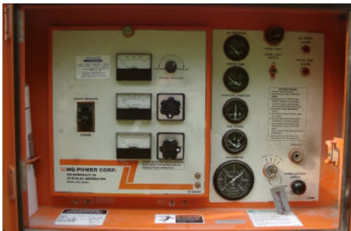
The "WhisperWatt" generator control panel. This is how power should be!
