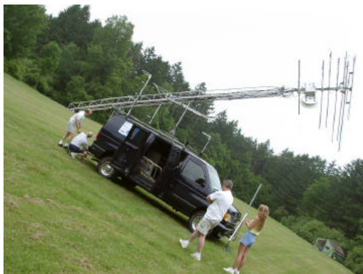
No, the earth didn't fall off it's axis. It's the only way I could get all the action in one photo. The N2JMH antenna array rises.
