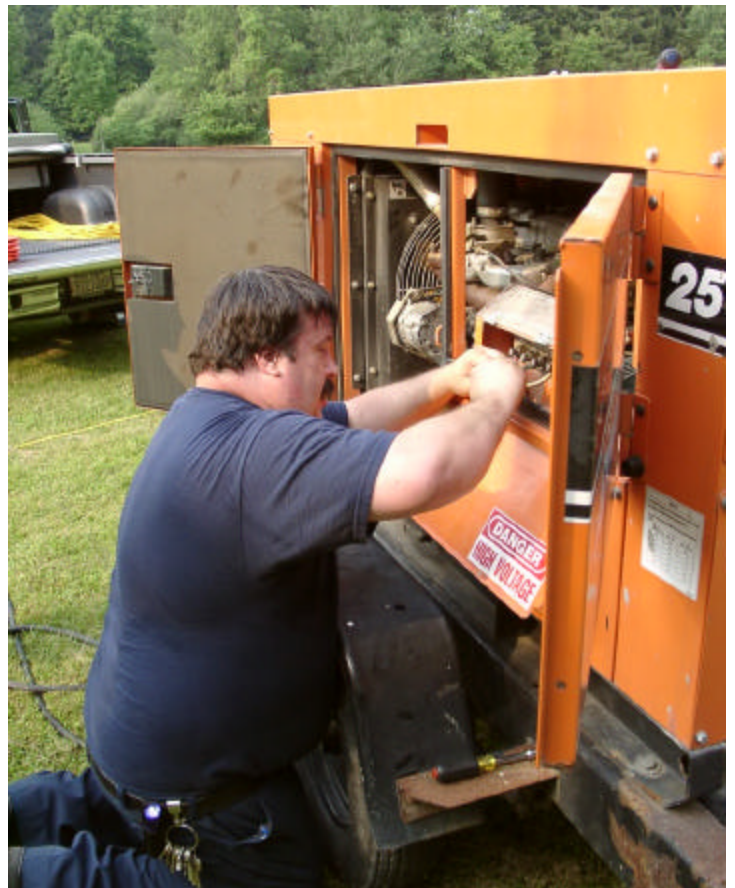
Power Arrives! N2QKL hooks up the main power line from the 25kW diesel generator, donated by Admar Supply Company.
