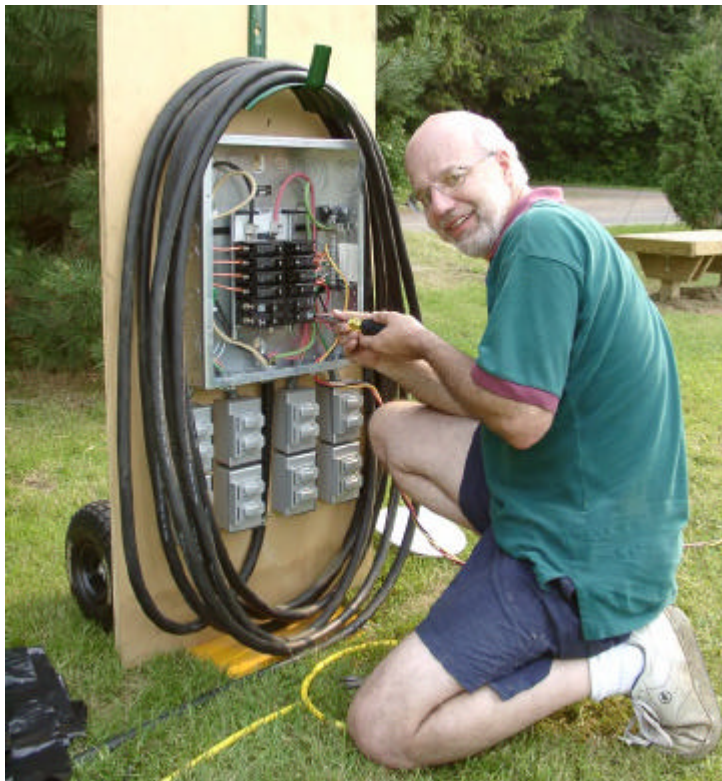
Electricity, just like at home! N2OPW wires in the 22VAC lines for the amplifiers. In addition to securing the generator, N2QKL supplied this distribution panel. Hookup was quite literally, just like home.
