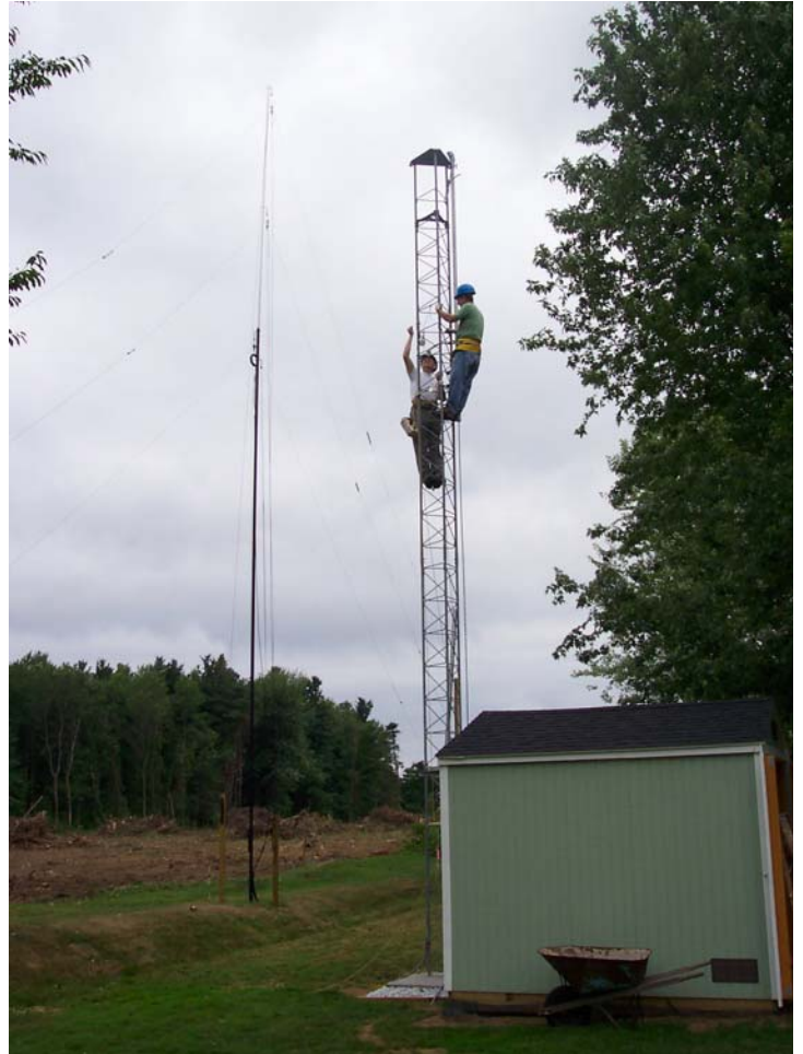
Bolting the top section of tower in place. The low band mast and VEEs are visible to the left of the tower.
