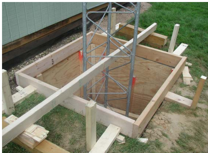
The hole, now dry, with the first sections of ROHN 45G installed and plumb.
