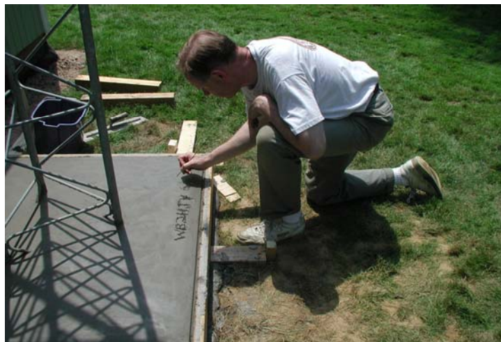
The finishing touch. No concrete pour is complete without a name and a date etched into the curing mass. WB2HJV does the honors.
