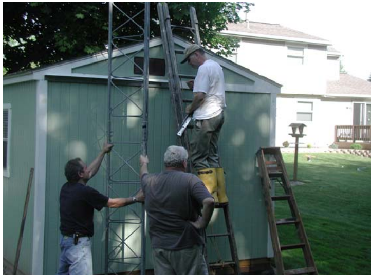
WB2HJV and friends erect the first two sections of tower and secure to the shed in preparation for the concrete pour.
