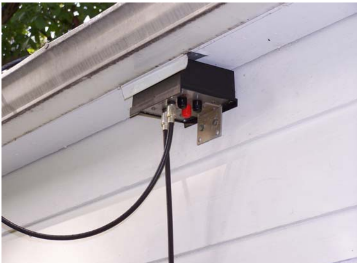
The Ameritron remote coax switch neatly mounted under the eave.
