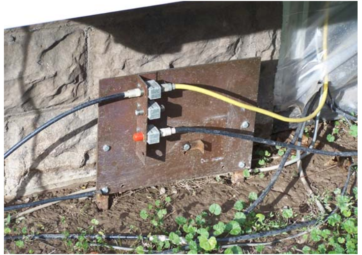
Grounding plate w/ 3 PolyPhasers mounted: one used for the tribander, one formerly used for the vertical and other antennas which were to be connected to the remote switch. Unfortunately, as Dave related in a previous article, PolyPhasers don't pass DC voltage, and he has currently bypassed the remote switch. Time to run a separate control cable, Dave.
