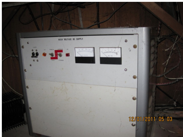
Power supply (under desk)
